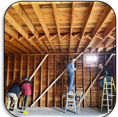
Bracing the building before it was moved. Jim Brady, Diana Brady, Chris King, and Austin Kiehl. Photo Credit: Laura Nowlin
